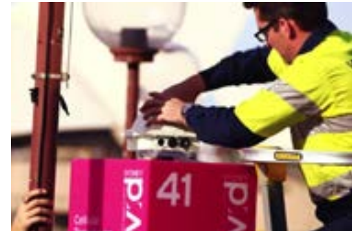
Figure 2: (Above) Ruckus ZoneFlex outdoor access points are installed upside down on the light boxes throughout the Vivid Light Walk, capturing the buzz of the event.
